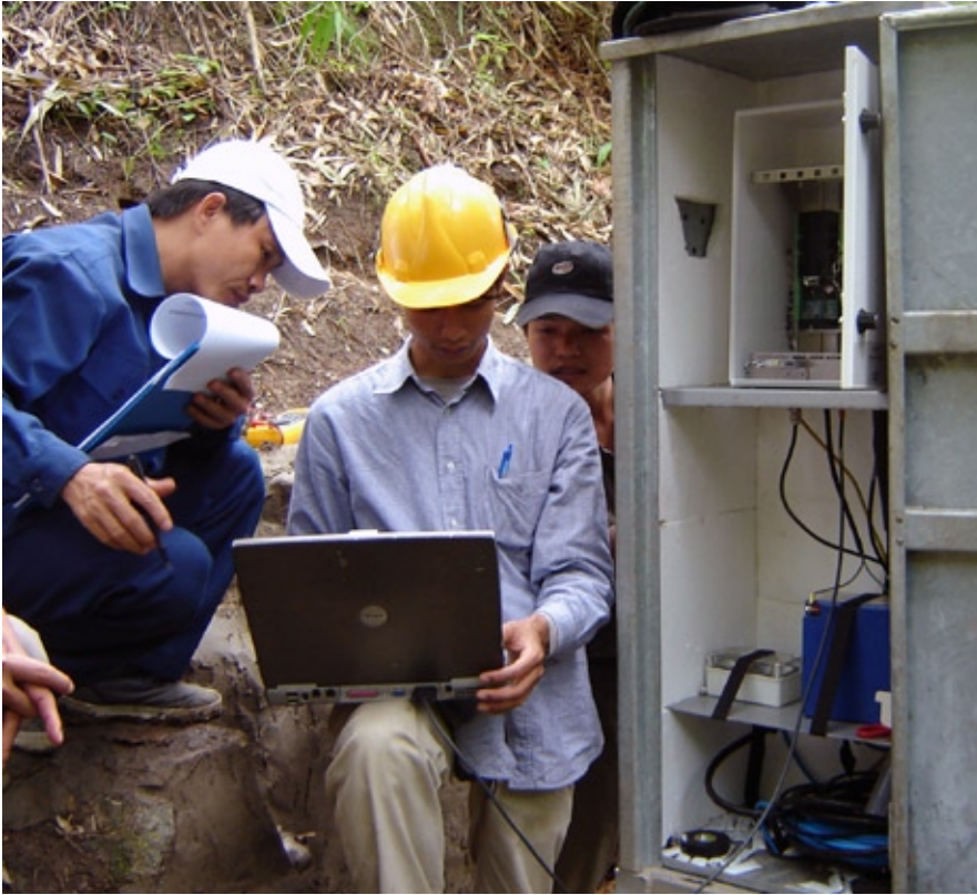
Site Acceptance Testing in progress.
